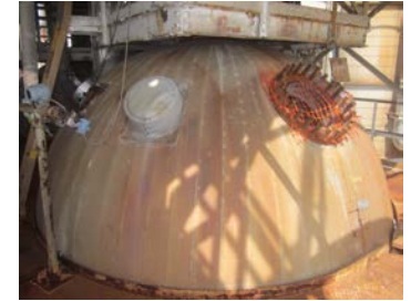
23,000 Gallon Reactor (One of Four) #103952
