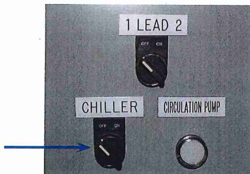
Single Circuit Chiller System
